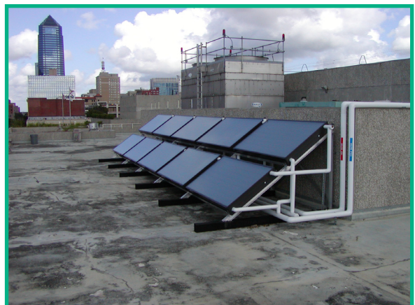
Commercial 10 PT50 rack installation
