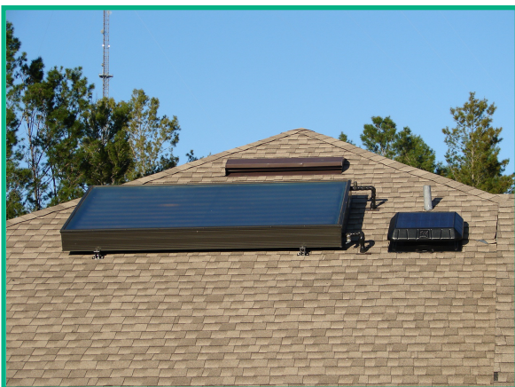
PT50 solar water heater and solar attic fan
